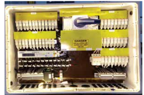
String Monitoring Box
