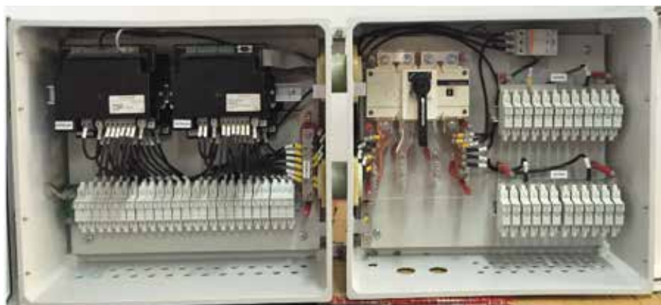
String Monitoring Twin Box
